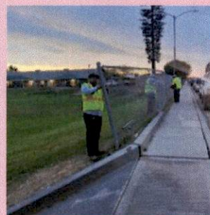
Damaged fence was remove at Las Villas.
